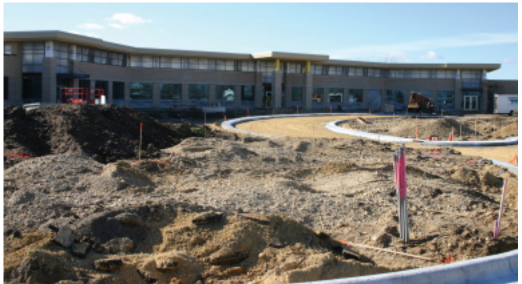
Blackhawk Technical College central campus is currently under construction. This shows what will be the new main entrance expected to be completed by end of next summer.
