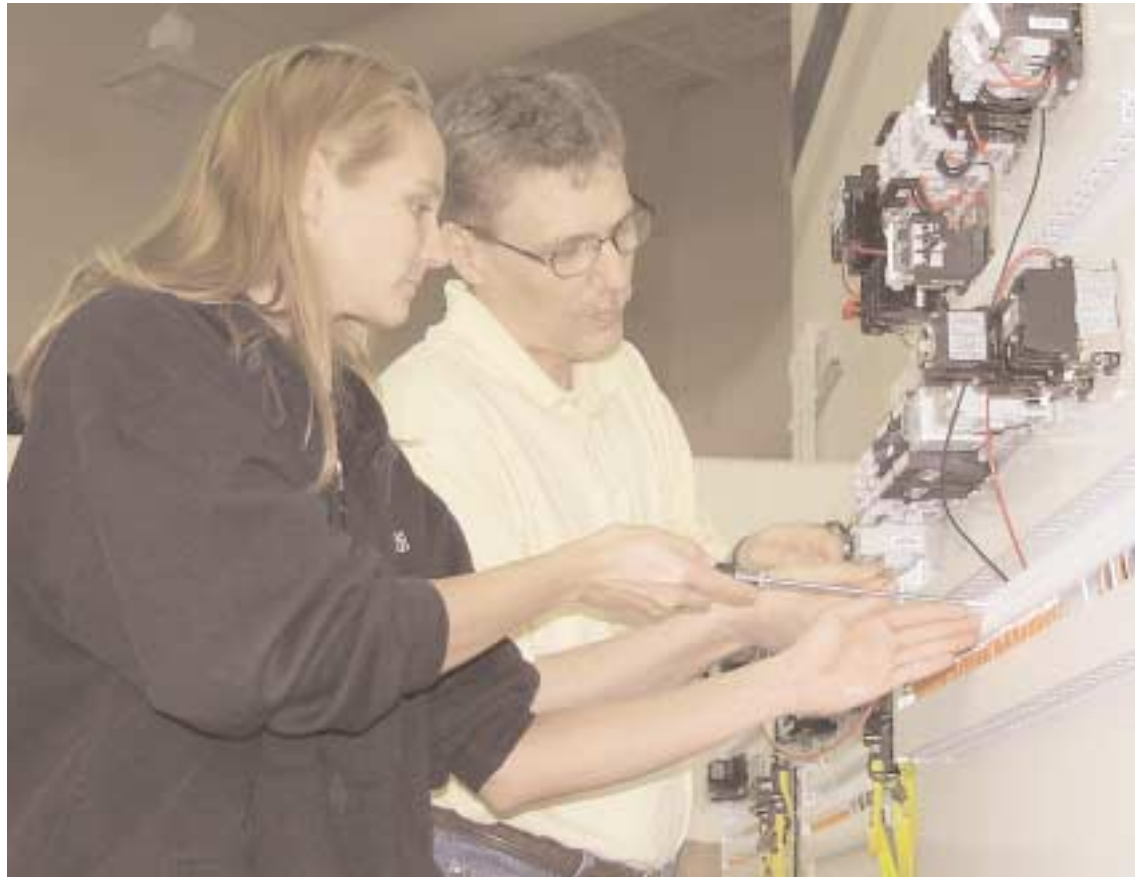
Large image above: Carrie Gottschalk and Mark Tilque, NWTC student apprentices, wire motor control circuits. In circle at right: Joe Messenger, NWTC student trains on Mecomtronics sensor application equipment . Small image at right: E&I Apprentice John Fournier programs on a PLC.
