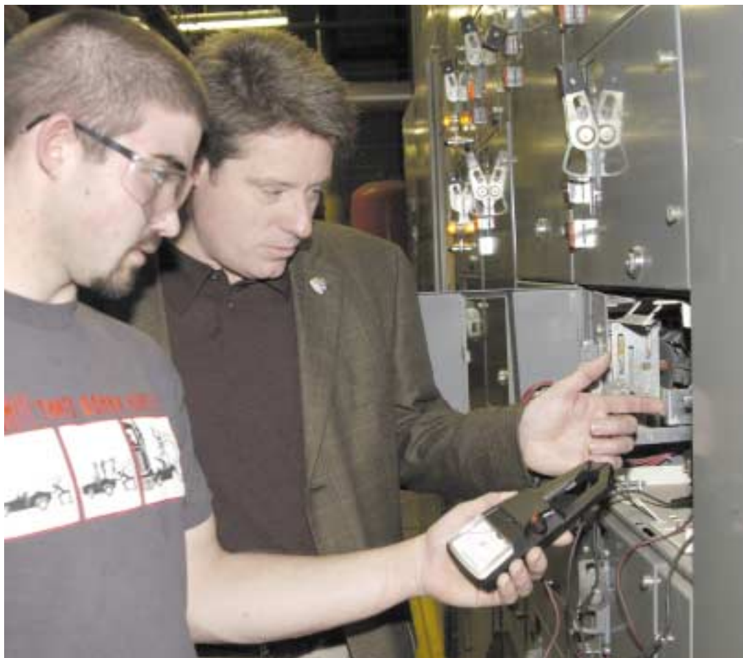
Power Engineering student Adrian Boldt runs a diagnostic test of boiler electrical controls with Mark Maierle, business manager of Local 317, International Union of Operating Engineers.
